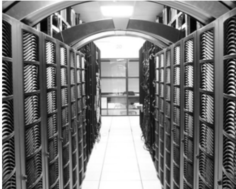
Data Center Build Out (photo by skreuzer, courtesy of Creative Commons).
