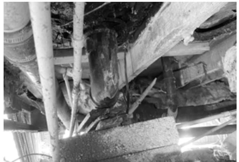
A busted sewage pipe causing a toilet to sink through the floor, being held up by cinderblocks (photo courtesy of Amory Fisher).
