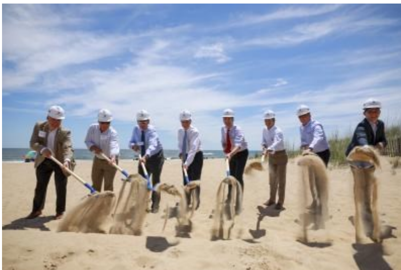
Pictured here: Governor Ralph Northam, other elected officials and stakeholders broke ground on July 1, 2019 at Camp Pendleton State Military Reservation in Virginia Beach to mark the beginning of onshore construction activities for the CVOW pilot project.
