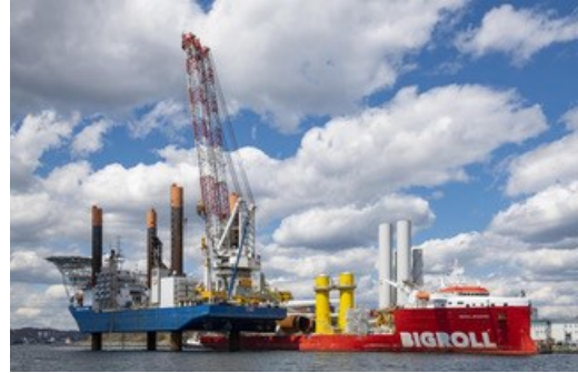
Photo credit: Dominion Energy
